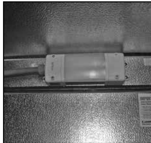
ABOVE DOOR LED LIGHT FIXTURE
