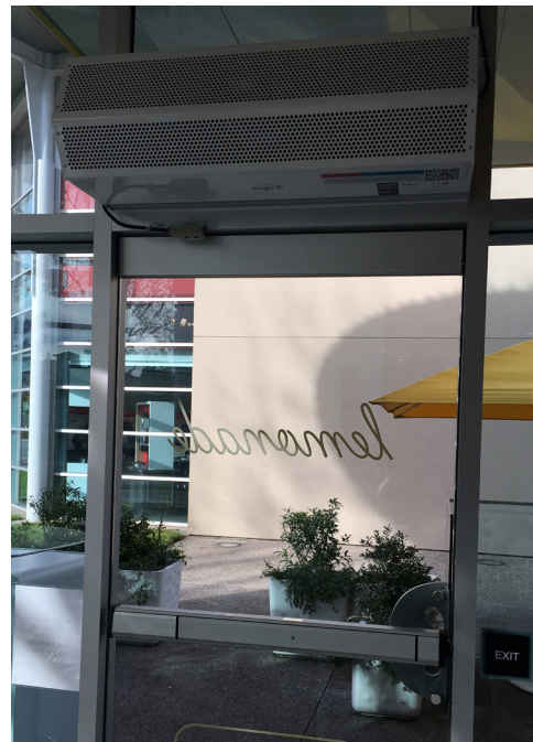
CUSTOMER FRONT ENTRANCES: The customer front entrance demands protection for superior cleanliness.
