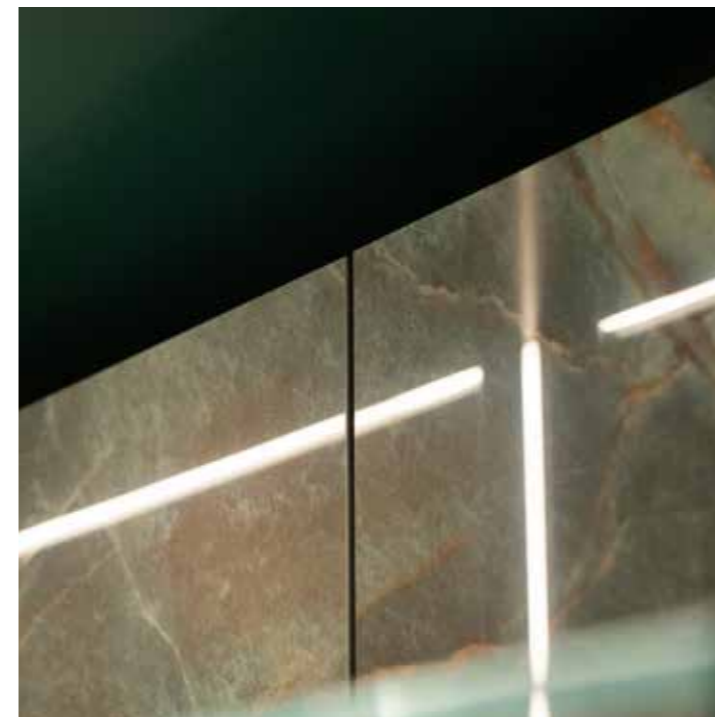
Air supply detail (top of the back panel)
