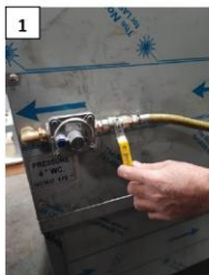
1 GAS VALVE IS CLOSED
